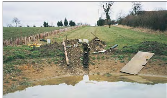
An agricultural field drain is intercepted and brought to the pond edge with pipework as a water supply
