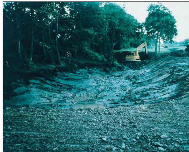
A 19th century origin Cheshire farm pond, used as a rubbish dump for thirty years, has been excavated in autumn, to its original shape
